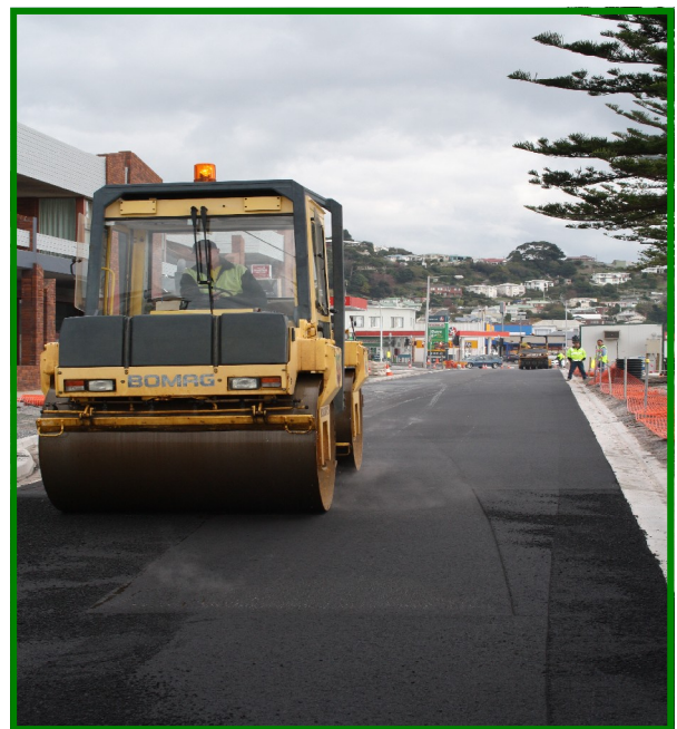
Sealing of North Terrace from Mount Street to east of Wilson Street.
