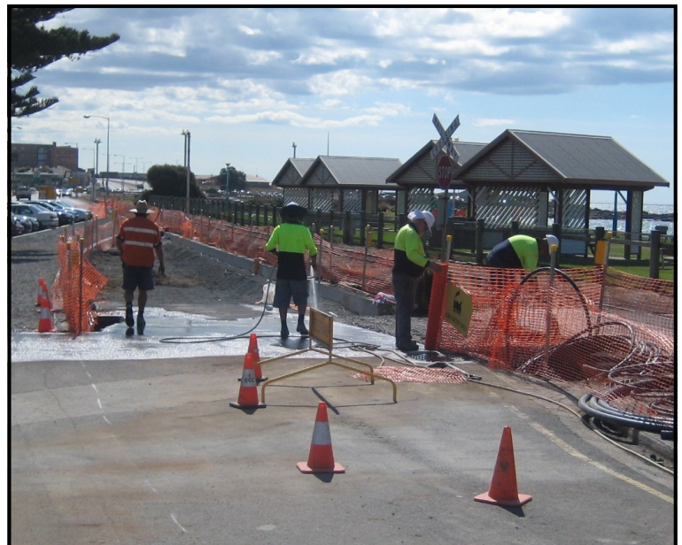
Council work crew with completed sections of rail fence plinth and garden bed surround.
