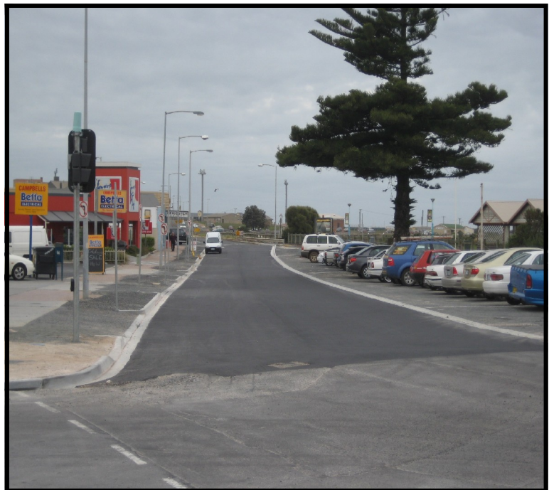
The completed kerb and channel and sealing works from Mount Street to Alexander Street 12 December 2008.
